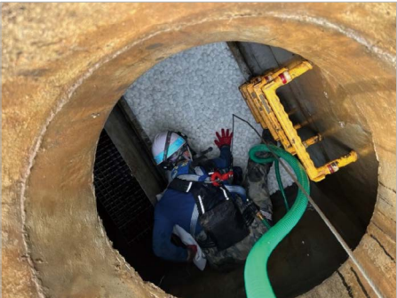
Filter replacement at non-point pollution reduction facility
